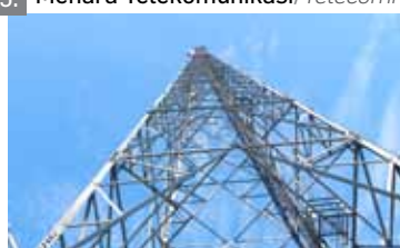
5. Menara Telekomunikasi/Telecommunication Tower
